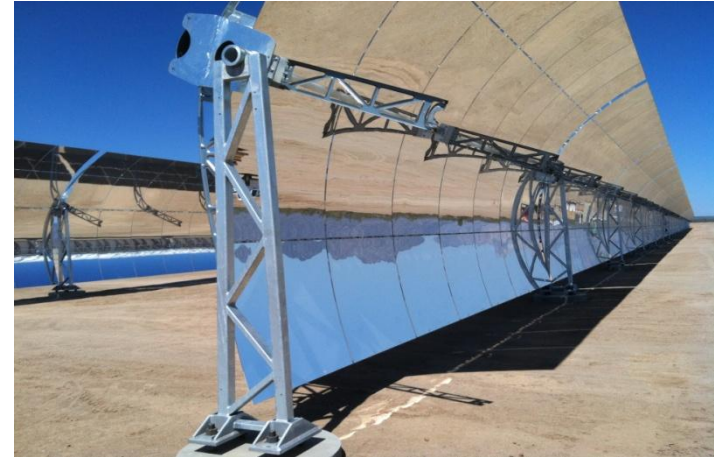
Solar Collection Assembly, Installed in the field
